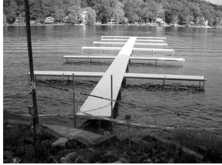
A "group pier" for 38 boat slips under construction. This is one of two 150-foot long piers proposed at this site on Lake James. However, an Administrative Law judge recently ruled that these piers were "unusually wide or long for the area" and don't qualify for a "General Permit." (Photo by Pete Hippensteel.)
