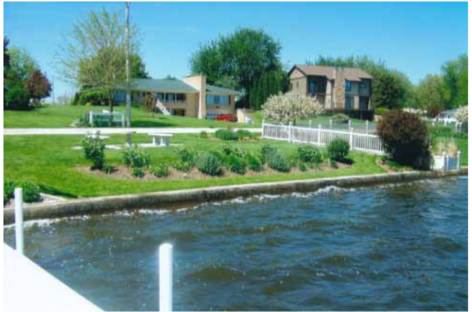
Figure 4. Seawall prior to re-facing with glacial stone.
